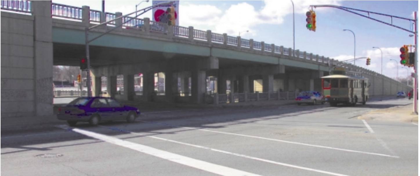
Many residents and leaders in Detroit and Ferndale, Michigan, want to see this Woodward Avenue bridge of Eight Mile Road demolished because it is a blight-inducing eyesore.
